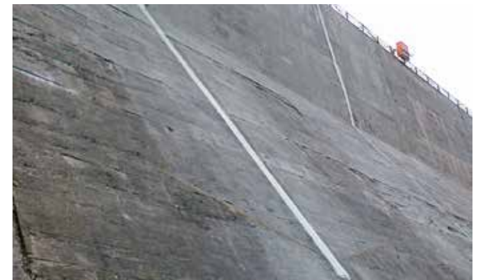
Relief cuts on dry side of Salanfe dam to reduce compressive stresses.
