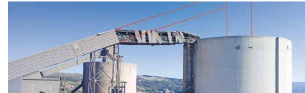
31 m diameter roof construction collapsed into silo together with filter and conveyor bridge.
