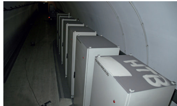
6 Soiling of the outside of the dust-proof switching cabinets
