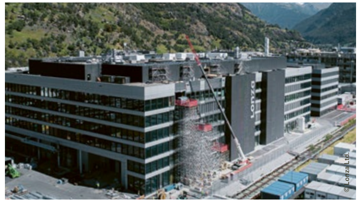
New Ibex® production building 106, Visp plant Client: Lonza AG, Basel Project period: 2017 to 2020 Employer/architect: Burckhardt+Partner AG Gruner services: Structural design, excavations, incl. bored pile foundations
