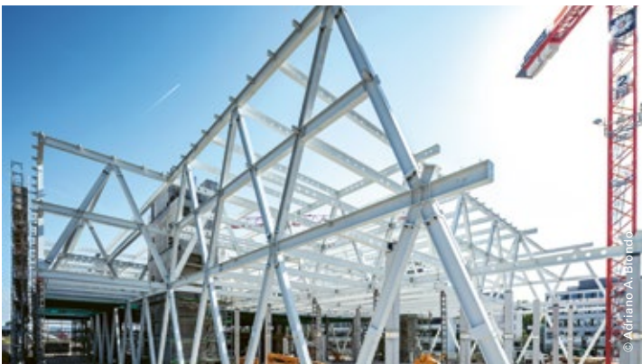
SKAN AG, new-build headquarters, Allschwil Client: Suva (Swiss Accident Insurance Fund), Lucerne Project period: 2018 to 2020 Employer/architect: Burckhardt+Partner AG Gruner services: Structural design for building and excavations, steel and concrete construction
